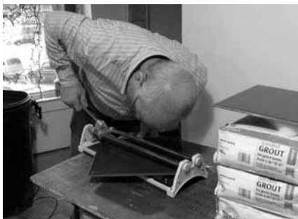
Snark Ron showed his construction background when he tackled the job of tiling the kitchen in the Hoo-Hoo House.
